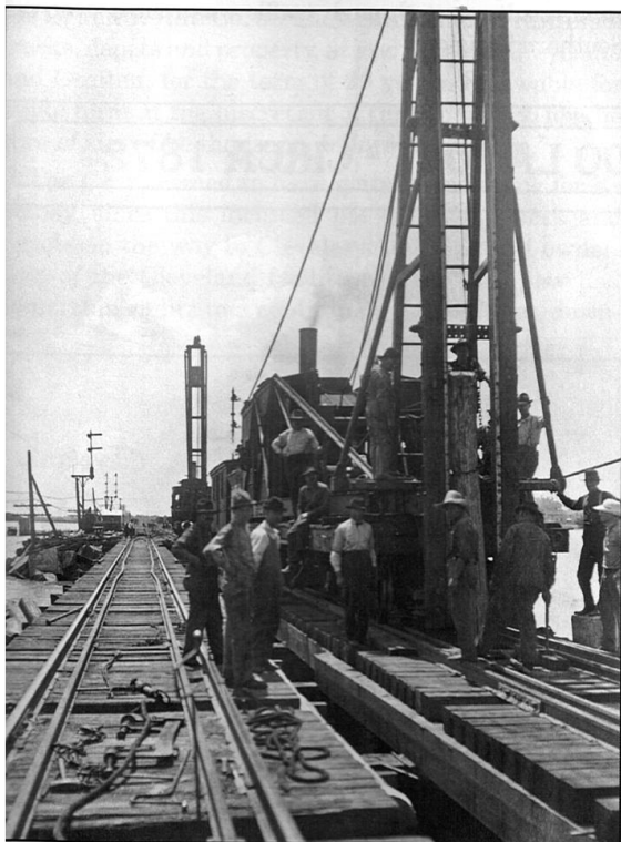
Sandusky Bay was the largest natural obstacle between Toledo and Cleveland. First bridged in 1855 by the C&T, then temporarily abandoned in 1858, the bridge was restored to service at the end of 1872 when the LS&MS rebuilt the track between Sandusky and Graytown. Here we see a pile driver and crew replacing pilings around 1910. Photo by Ernst Niebergall. Charles E. Frohman Collection/Hayes Presidential Center.
