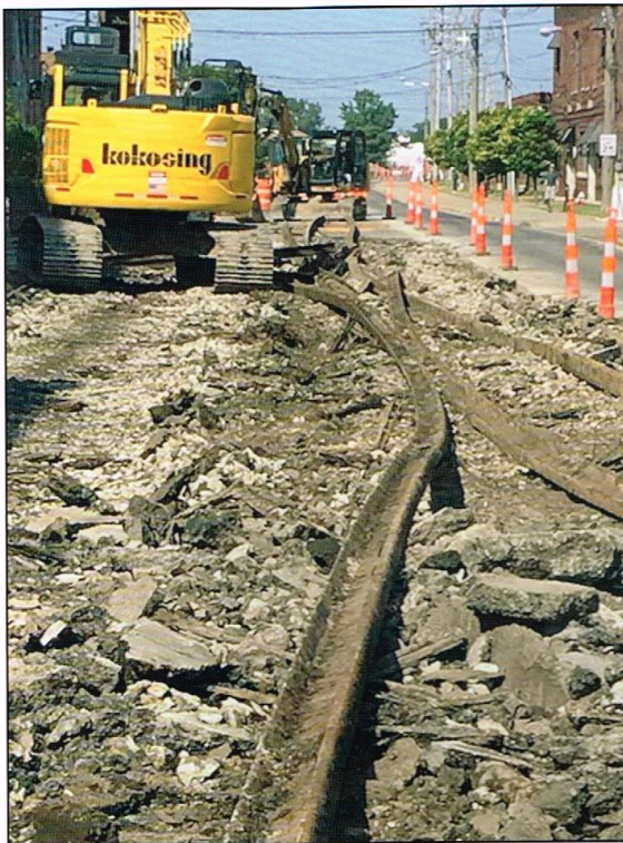
While Railroad Street has long been renamed Shoreline Drive, the pier tracks still remained, although paved over. During the end of June and beginning of July 2019, the buried tracks were being removed, ending their nearly one-hundred-and-seventy-year presence. Photo by the author.
